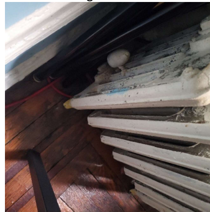
Figure 4.2.2 Air vent on Existing Radiator
