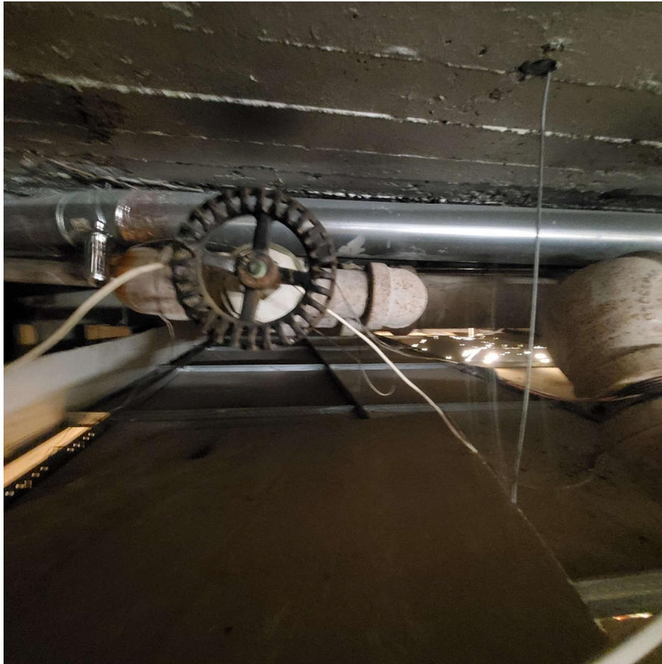
Fig. 9.5.2 Master Steam Vent in Office @ [REDACTED]
