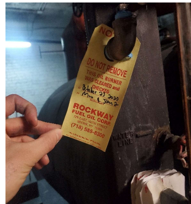
Figure 3.2.4 Burner Inspection Tag
