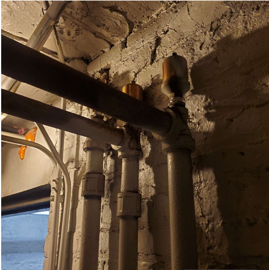
Fig. 9.5.1 Master Steam Vents in Boiler Room @ [REDACTED]
